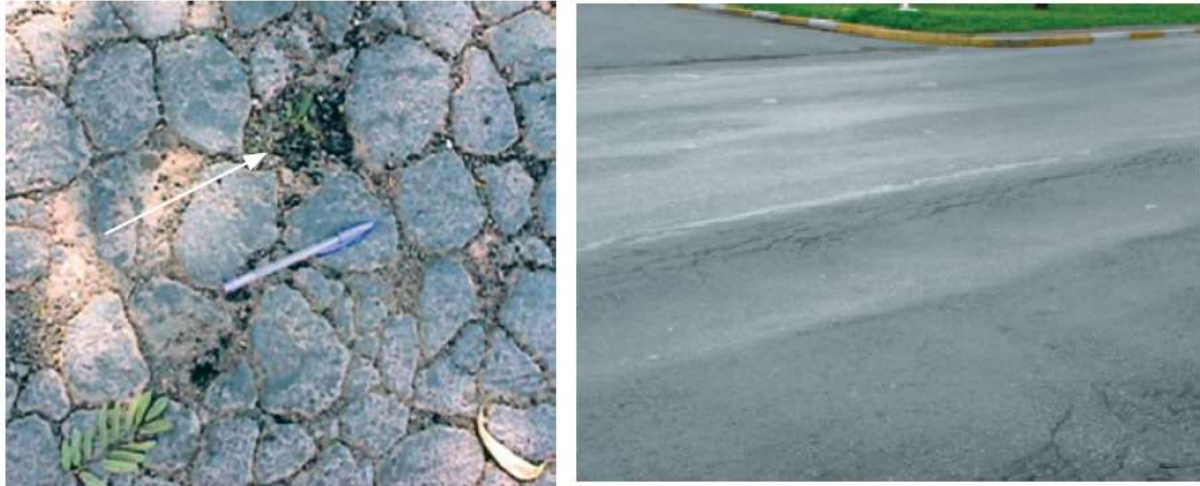
FIGURE 2 - (A) MACROCRACKS FORMED DUE TO EXCESSIVE FATIGUE CRACKING (B) PERMANENT DEFORMATION.
