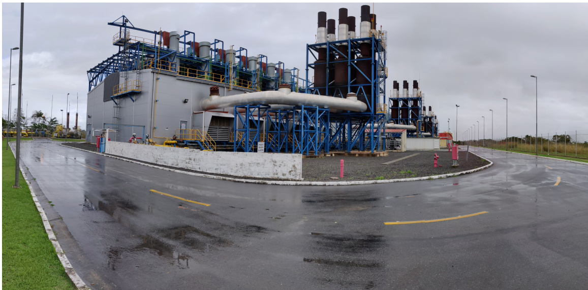
Figure 1 – UTE LORM thermal power plant.
