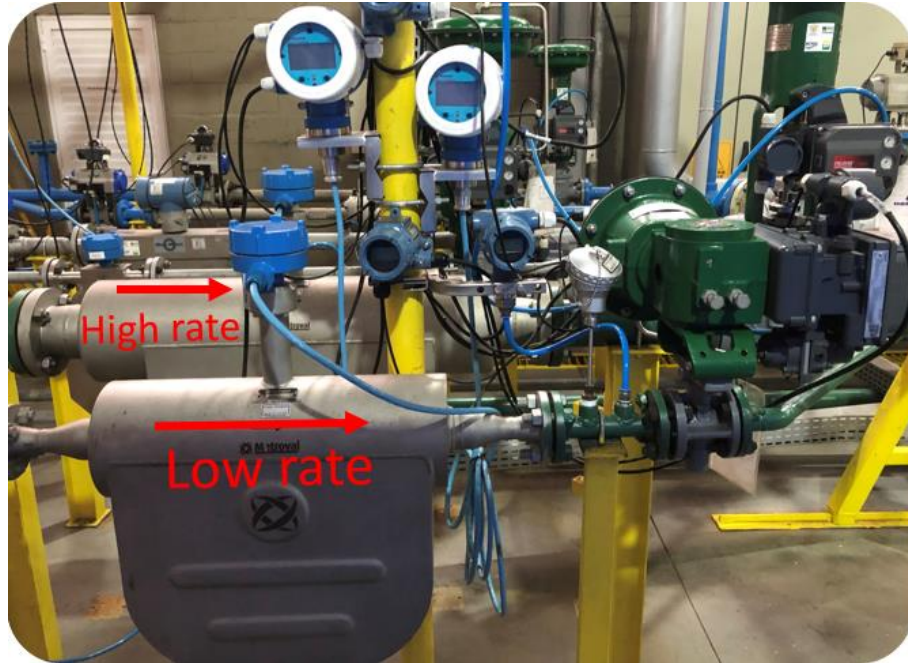
Figure 21 - High and low waterflow rate Coriolis meters in split-range arrangement photography (Source: author)
