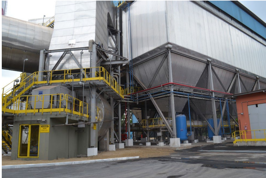
Figura 6 – Gas Cleaning Bag Filter.
